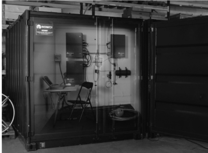
Figure 2. Automatic monitoring station.
